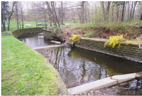
PHOTO ABOVE: Downstream (north) of Wade Park Avenue, in-channel concrete barriers and failed wall will be removed and the channel reconstructed similar to the schematic, shown below.
