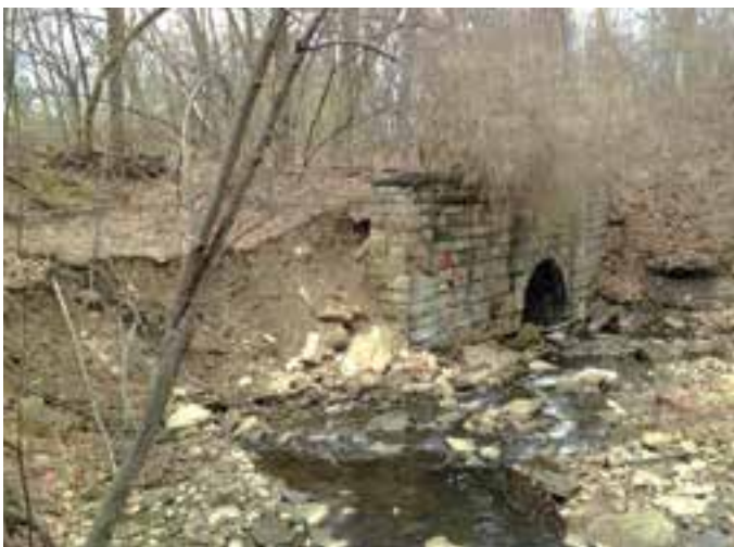
Erosion as a result of the failed debris rack.
